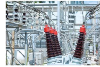
Transmission, Distribution, and Substation
