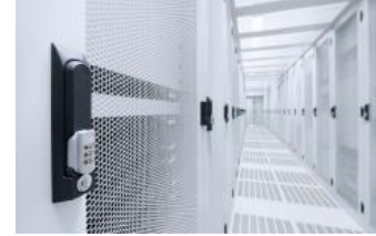
MTDC and Colocation Facilities
