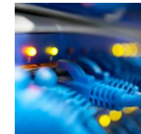
Network Infrastructure and Security
