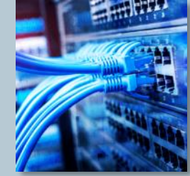
Network Infrastructure and Security
