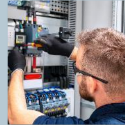
Electrical Distribution and Controls
